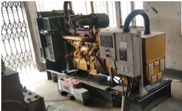
Pic 9: Standby Power Generator Facilities
