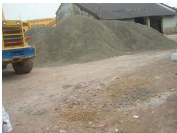
Pic 36: Loose Material Placed next to the Road
